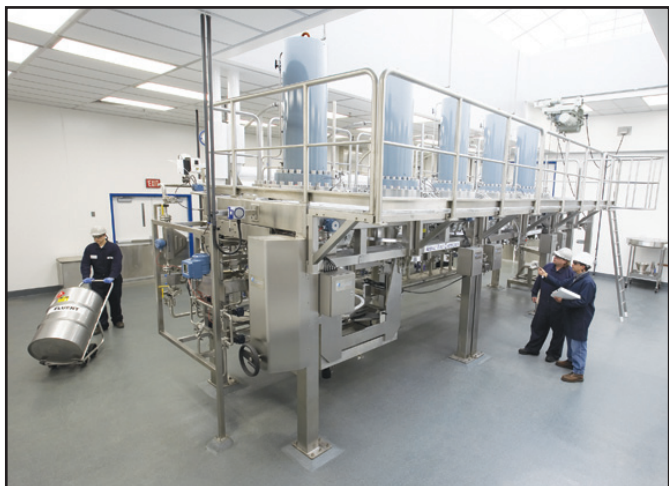
The 5x1000mm SMB unit installed in 2006 is the largest of the 6 units installed at AFC to provide separation services from gram to multi-tonne quantities.
